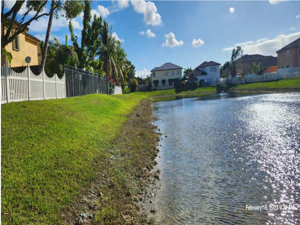
Figure 16: Bank Erosion with soil repose itself and at the same time slope become steeper
