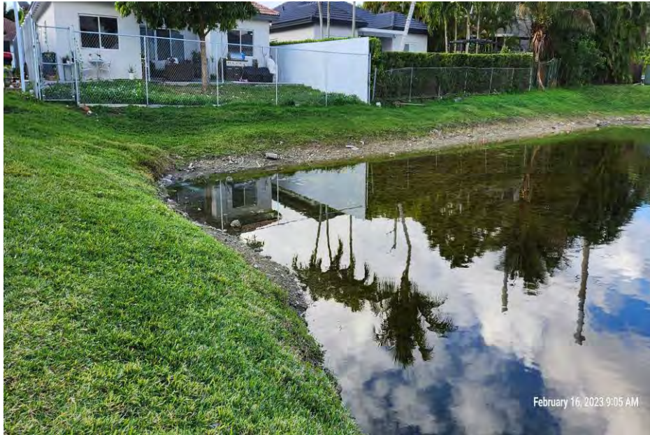
Figure 12: Bank Erosion with steep drop and unstable embankment.
