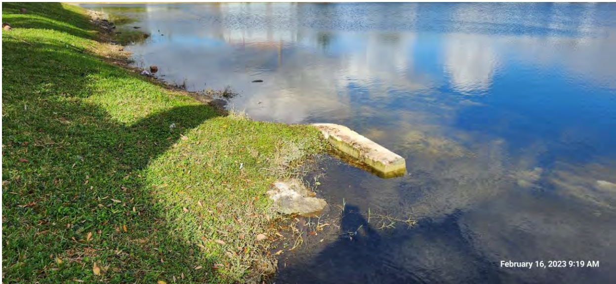
Figure 13: Bank Erosion shown lost soil over the years
