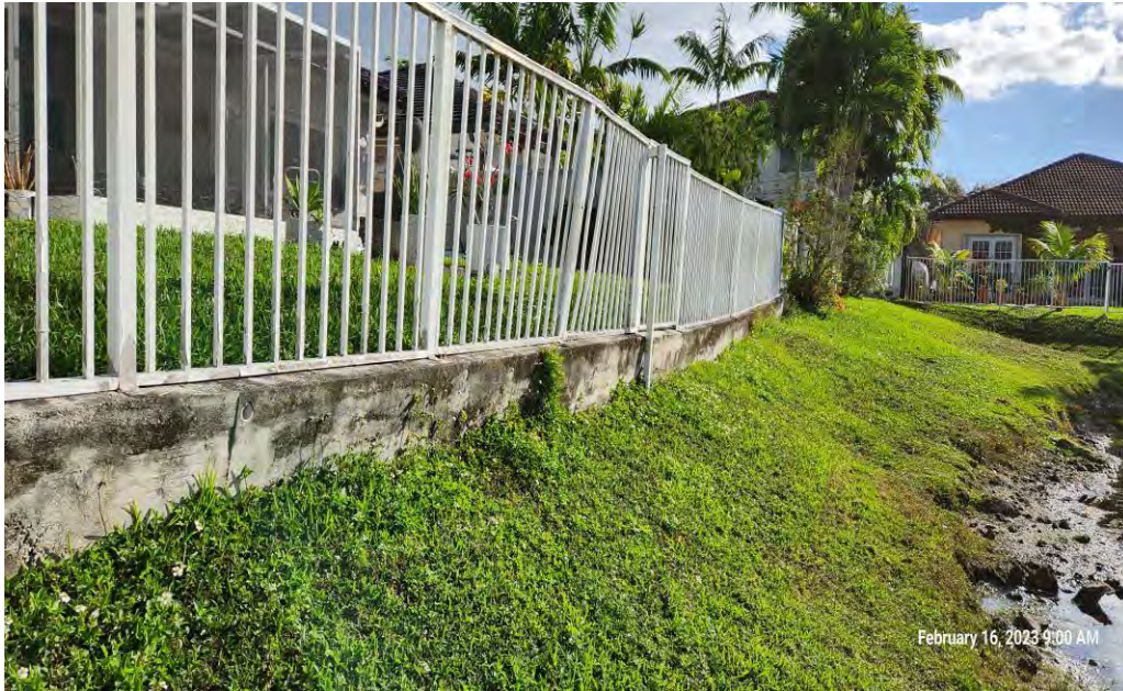
Figure 7: Retaining wall failed, because of unsettled soils and saturated soils that increased the hydrostatic pressure.
