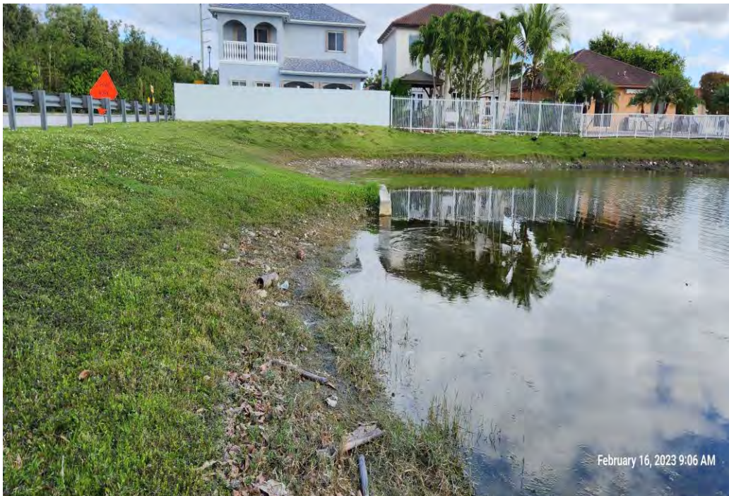
Figure 8: Bank erosion, shown lost land and reposed embankment.
